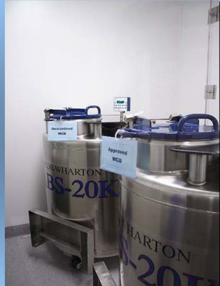
LN2 Tank for WCB Storage
